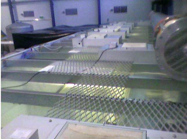
Figure 3: Air filters on laser enclosure; filter 9 at front.
