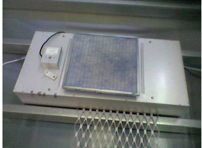
Figure 4: Filter 1 on the laser enclosure
